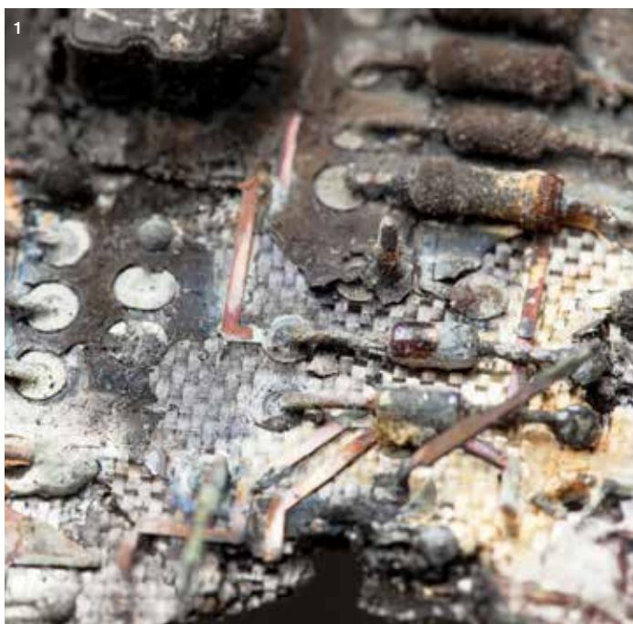
1 Transient overvoltage damage to a circuit board | 2 Most damage is barely visible
